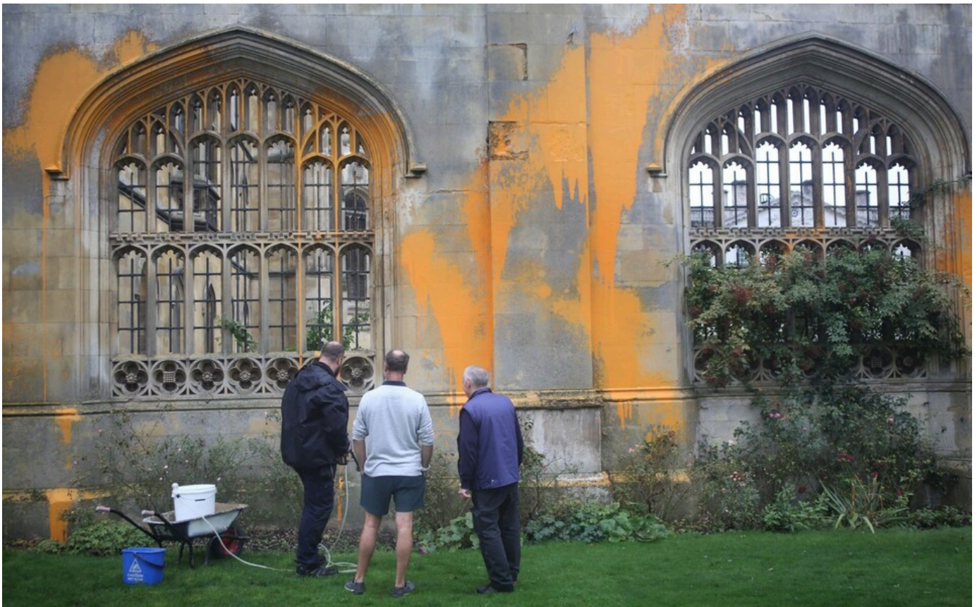
University staff inspect damage to the exterior of a 15th century King's College building from climate protesters. Credit: Martin Pope/Getty Images
