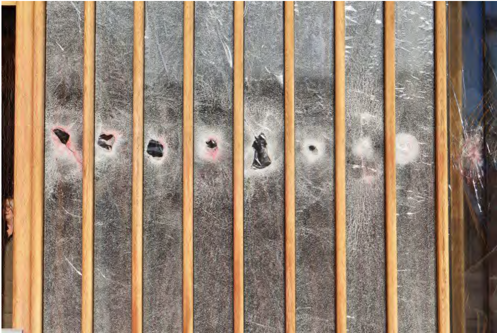
Broken windows at the front entrance of the Blavatnik School of Government. Credit: Kate Bansmer
